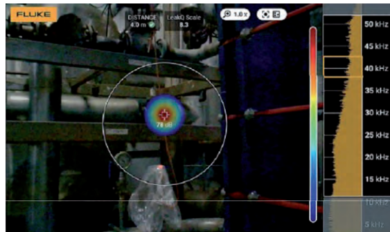
Steam leak captured with the Fluke ii910 in a food and beverage manufacturing plant
