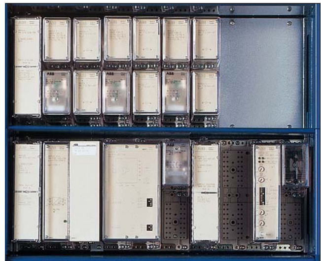
Picture showing some of the Static Protective Relays in the Power Plant Module.
